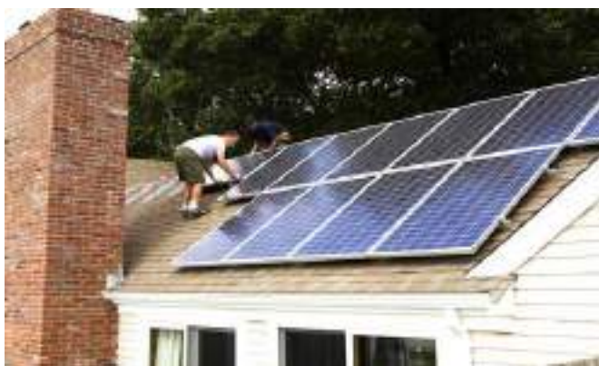
Fig 8. Building Attached Photo Voltaics
