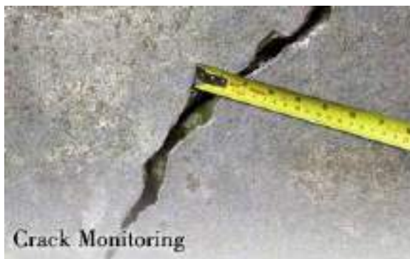
Fig. 1. Monitoring cracks using tape and pencil
